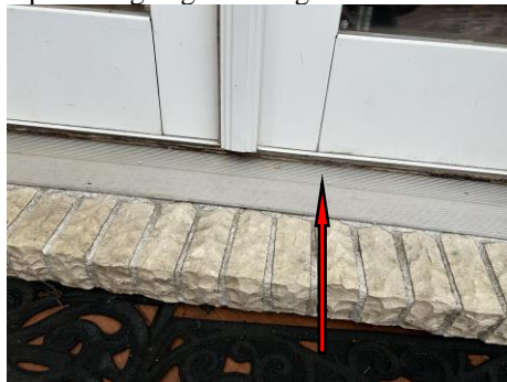
Rotten wood under doors to deck.
