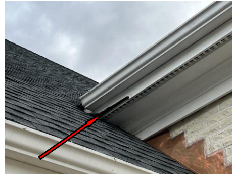
Damaged fascia front center area.
