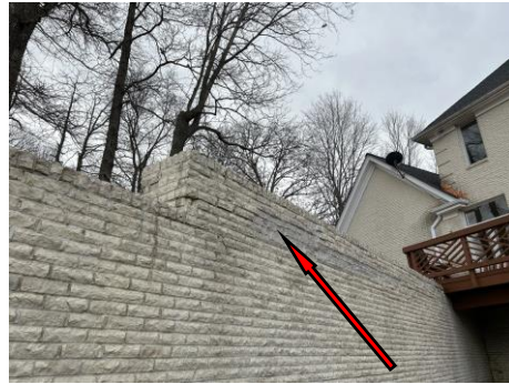
Right side rear retaining wall damaged at the top
