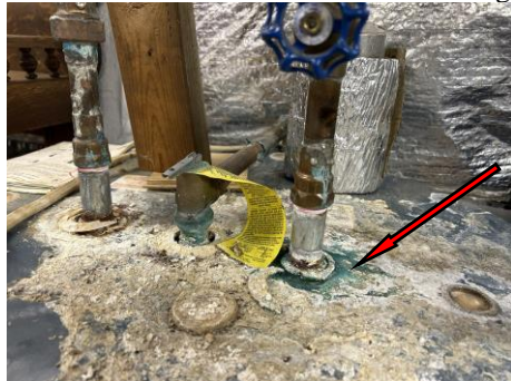
Leak on top of water heater.
