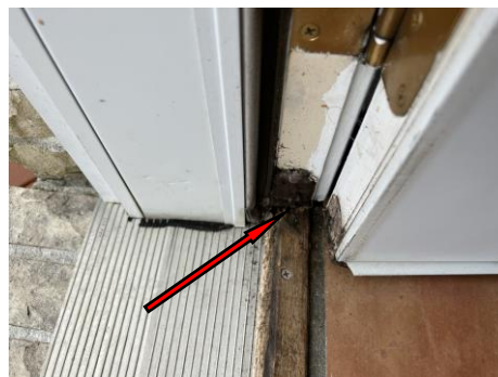
Rotten thresholds doors to deck.
