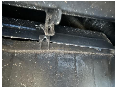
Living room damper off track.
