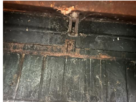
Master bed damper missing handle.
