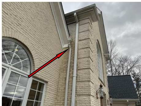
Gutter left of front door appears to leak onto house.
