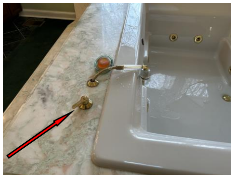
Master bath wand selector knob not working.
