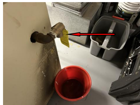
Pressure relief valve on boiler leaking.
