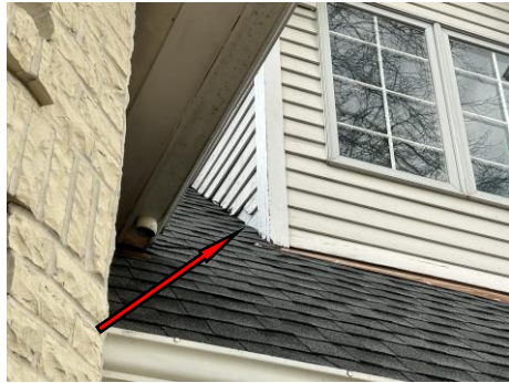
Missing siding front left dormer.
