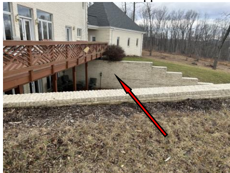
Hand rail on top of retaining wall?
