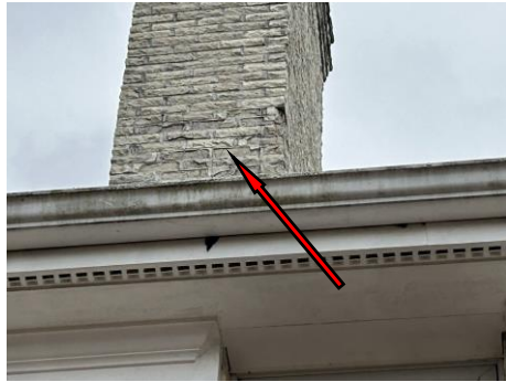
Spalling bricks back side of center chimney.
